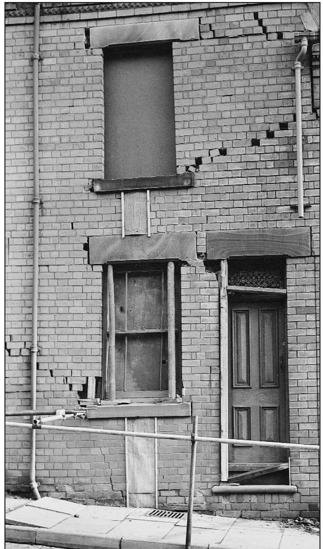
Figure 7. Damage to a terraced house in Belvoir Street, Hucknall, in 1955. The house has since been rebuilt.
