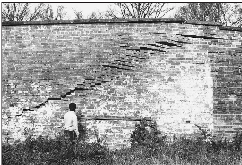
Figure 1. Reactivation of a fault generated a 0.3m high fault scarp and caused severe damage to a 5m high brick wall at Eastwood Hall. The date of reactivation is not known, but was probably in the 1960s. This section of wall has been demolished, but evidence of further fault reactivation was visible on an opposing wall in May 2000.
